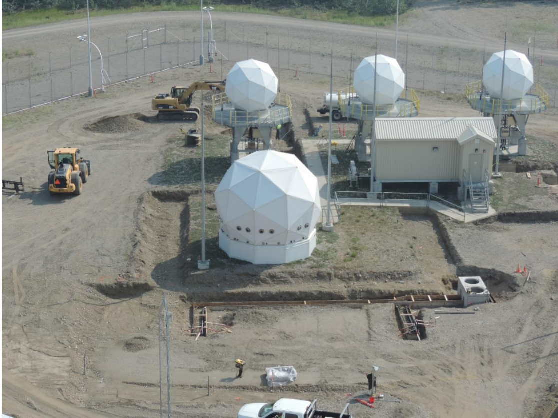
EPS/EP-R Gateway Site construction at Clear SFS on Wednesday, 29 June 2022. (U.S. Space Force photo: Lacey King).
