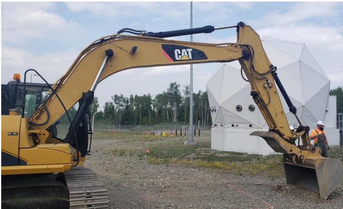
EPS/EP-R Gateway Site first shovel at Clear SFS on Thursday, 23 June 2022. (U.S. Space Force photo: Lacey King).
